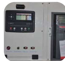
Control Panel & MCB
